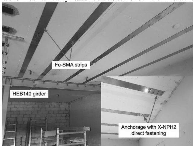
Figure 1 Re-plates (Fe-SMA strips) are installed as pre-stressed strengthening elements for a reinforced concrete slab [Michels et al. (2018)]
