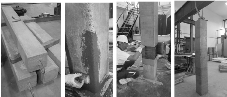
Figure 2: Preparing the surface of the columns (2400 mm), round of corners and applying CFRP strengthening.
