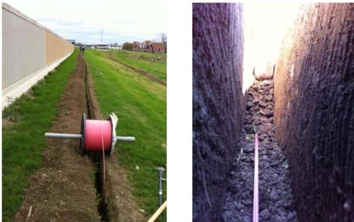
Figure 5. Installation of SMARTprofile sensor in a trench on the surrounding of the levee wall.
