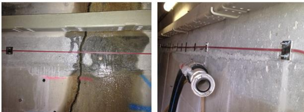
Figure 11 SMARTprofile sensor installation on penstock access tunnel.
