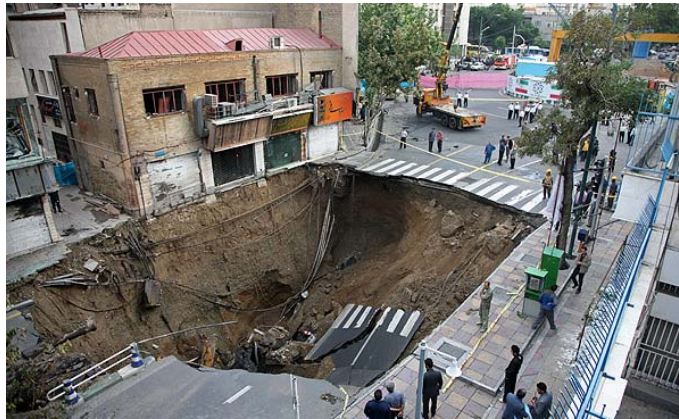
Figure 3. Collapse of the street at F3 station located in the next crossroad of D3L7 station.
