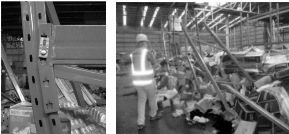
Figure 2. Collapsed rack system in Christchurch earthquake in 2011 (Clifton et al. (2011))
