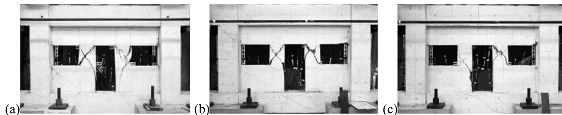
Figure 5. Crack patterns at first full cycle to 1% drift: (a) B-WOA; (b) BH-WOA-V, and (c) BH-WOA-VH
