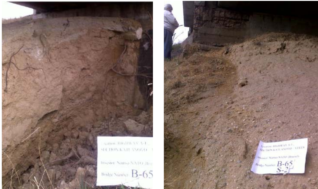
Figure 2. View of eroded ravine in front of abutments S-1 (left) and S-2 (right) on bridge B65
