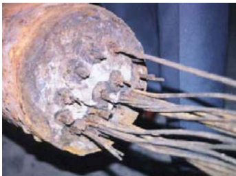
Figure 4. Load side of a socket that failed. Most steel strands broke, mainly due to corrosion, in the vicinity of the socket.
