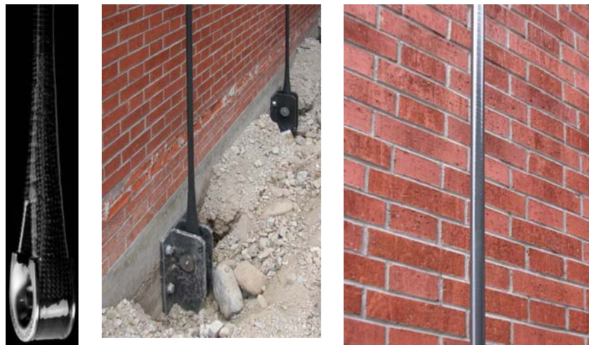
Figure 11. Seismic retrofitting of a masonry wall post-tensioned with a pin-loaded CFRP strap system. Left picture: termination for pin-loading. Middle picture: Attachment of the CFRP strap to the concrete foundation with pin-loading. Right picture: Post-tensioned CFRP tendon of 1 MN load capacity.
