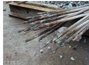
Figure 6. Some wires of the strands show brittle fracture surfaces probably due to corrosion, fatigue and fretting.
