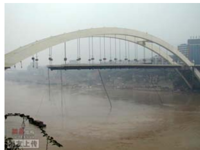
Figure 3. Xiao-nan-men Bridge with collapsed bridge deck.
