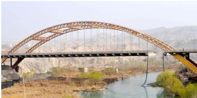
Figure 7. Kong-que-he Bridge after failure in 2011.
