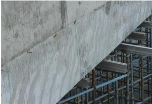
Figure 5. Diagonal shear cracks on the Western edge at the NW corner
