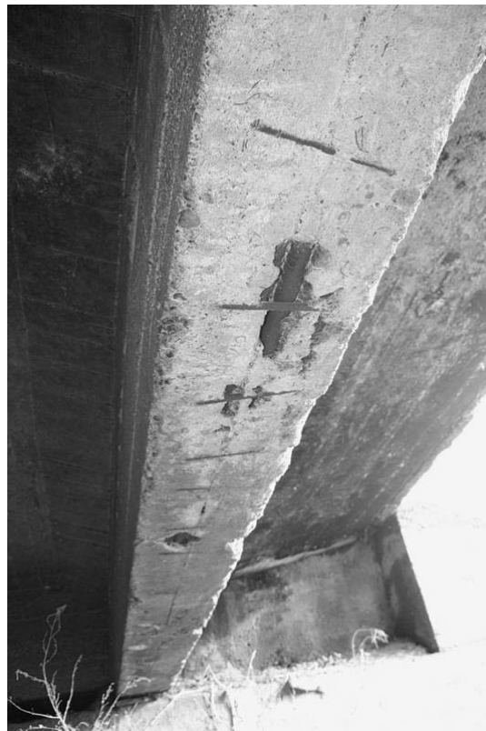
Figure 4. Exposure of reinforcement under a beam due to construction defects (inadequate cover depth).
