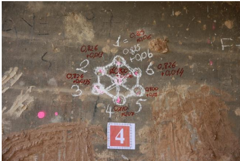
Figure 4. Application of Windsor pin test on vertices and center of a hexagonal marking drawn on a bridge pier wall. Measurements at each point are written on the bridge member and photographed.
