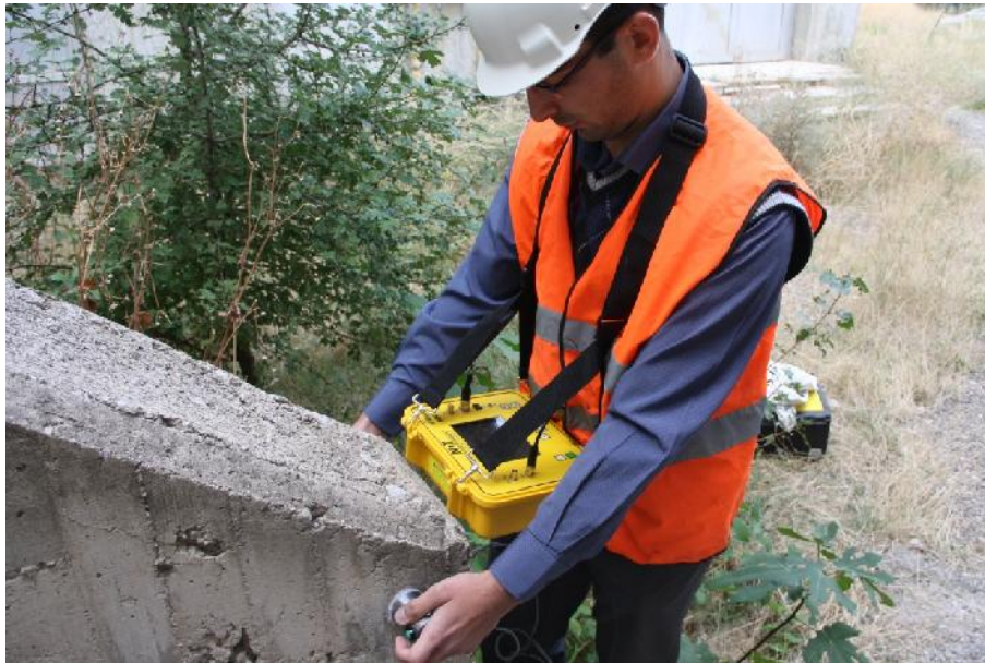
Figure 2. Application of ultrasound pulse velocity device on a concrete bridge wing wall.
