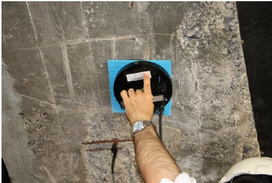
Figure 3. Application of reinforcement corrosion resistivity (corrosion rate) device on a reinforced concrete bridge girder.
