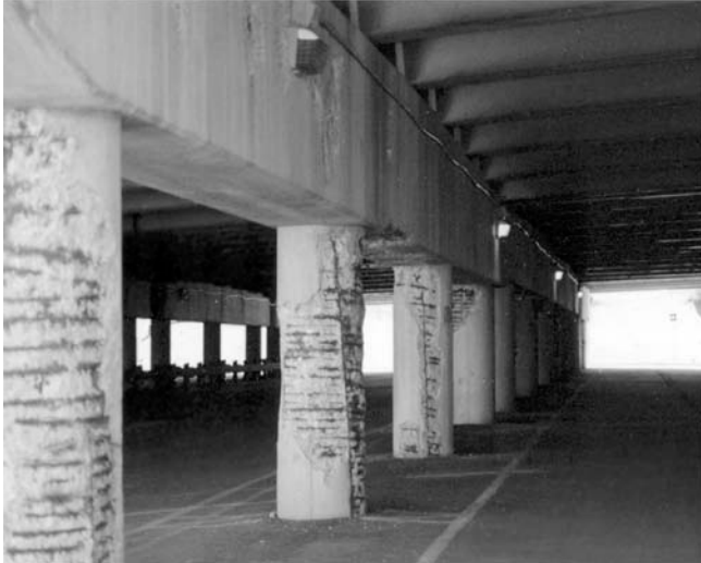
Figure 1. Corrosively damaged bridge columns.
