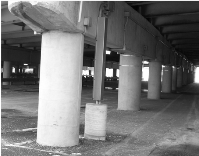
Figure 6. Repaired columns after fifteen years of service.
