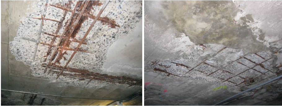
Figure 2. Corrosion of steel reinforcement of in parking garage.
