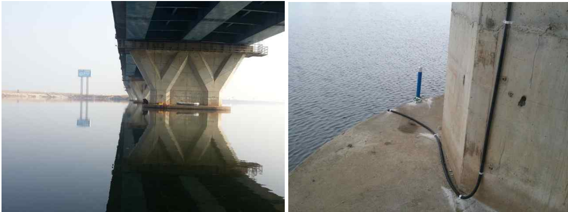
Figure 5. Measurement surroundings and the installed instrument in the river
