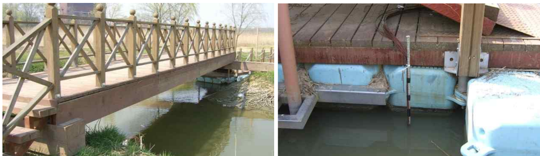
Figure 2. Measurement surroundings and the installed instrument in a stream
