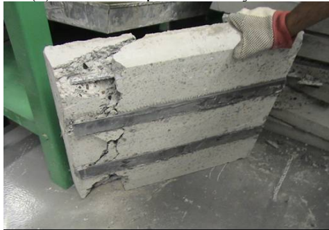
(c) typical slab failure (bottom view)
