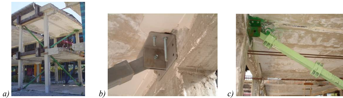
Figure 9. The RC structure equipped with BRBs: global view (a) and zoom in to the BRB 1 (b) and 2 (c).
