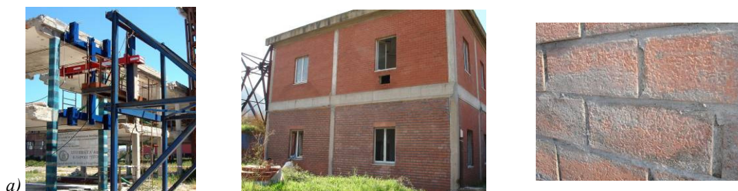
Figure 3. The C-FRP repairing/upgrading systems: a) building No. 1; b) and c) building No. 2.
