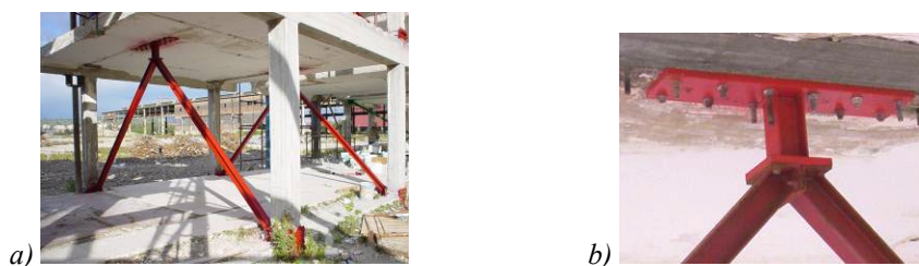
Figure 7. The RC structure equipped with eccentric braces: global view (a) and zoom in to the link (b).
