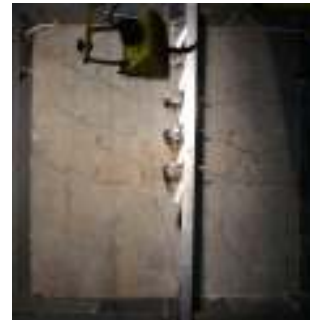
Figure 2 Crack Pattern of the Reinforced Concrete Slab
